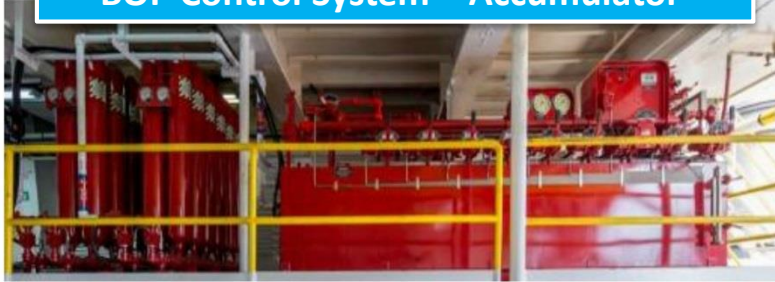
BOP Control System – Accumulator
